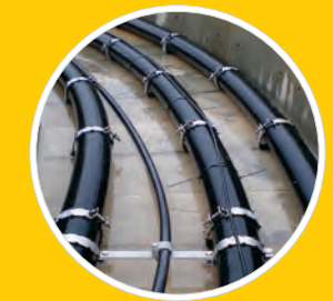
Underground Electricity with Transformer
