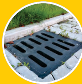
Underground Drainage System
